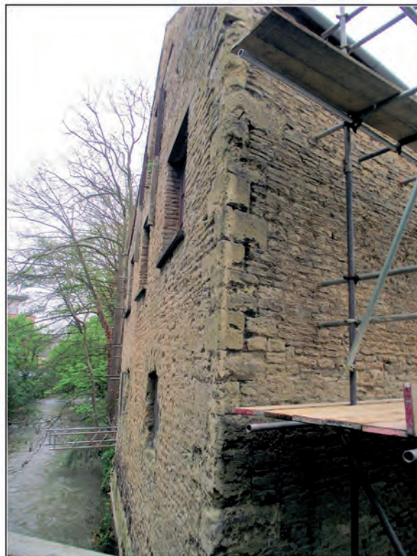
Fig. 14. The Old (or Paradise) Malthouse in 2014, showing the river frontage and the sharply angled south-west corner.
