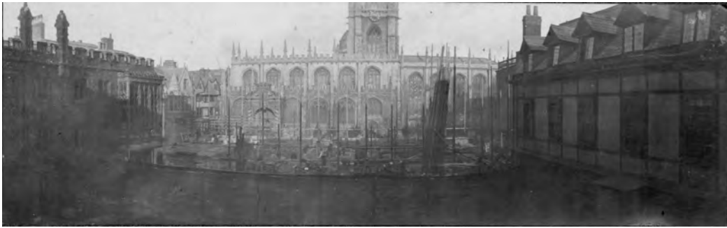
Fig. 3. The Rhodes Building under construction, as viewed from St Mary's Quad. The High Street and the front of St Mary's church can be seen through the forest of poles (OCA, FB 5 B3/2).
